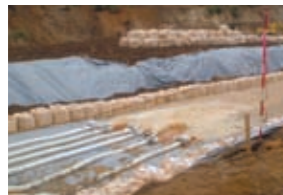
KUBOTA installed movable pumps to pump out water and prevent a secondary disaster.
