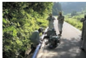
Urgently needed temporary water pipes were laid to supply water to the area affected by the water outage.
