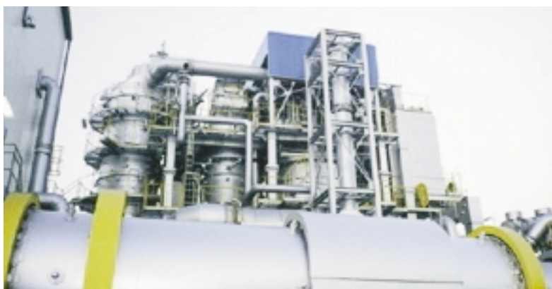
Pyrolysis melting furnace
