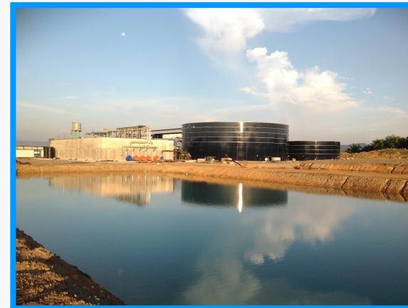
Effluent treatment and biogas recovery system for palm oil plant in Malaysia (Under construction)
